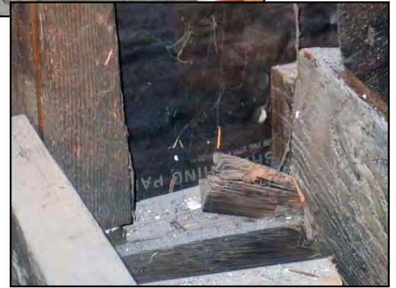
Ceiling truss severely compromised.
