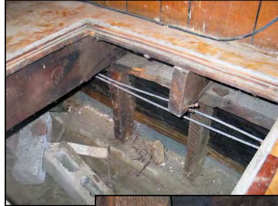
Severe termite damage at the foundation.
